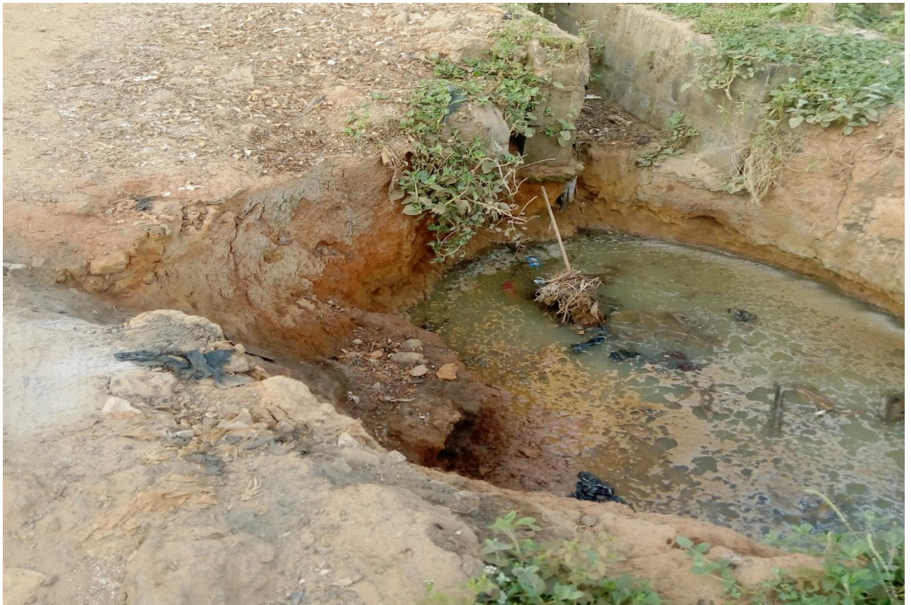
Picture 9: Eroded Portion of the Omadewu road, caused by the effluents.
